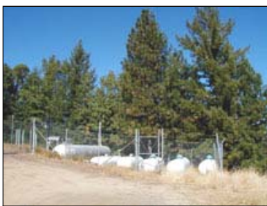
South Hoadley Peak propane tanks for the communications facility.
