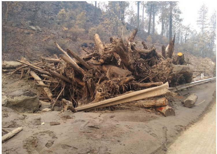
Debris flow piled against a bridge on Little Humbug Creek, a tributary to the Klamath River, during the 2022 McKinney Fire. Photo by E. Peterson
