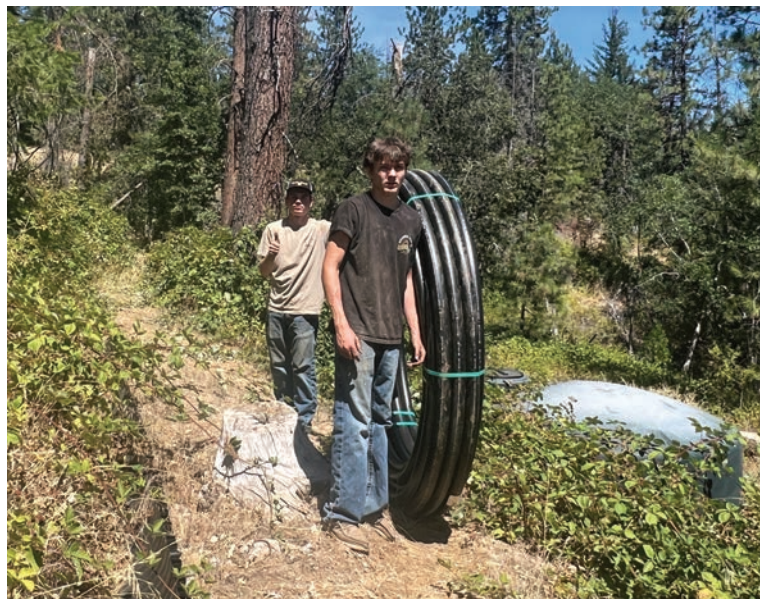
Jack Proburko and Kenny Plew support their grandfather Rod Plew by hauling rolls of pipe along the ditch line to the next installation site
