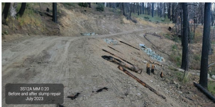
Slump Repair on the 3S12A Rd., Horse Ridge, Six Rivers National Forest
