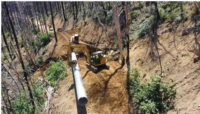
Culvert Replacement on the 28N10 Rd. at Beegum Creek, South Fork of the Trinity River
