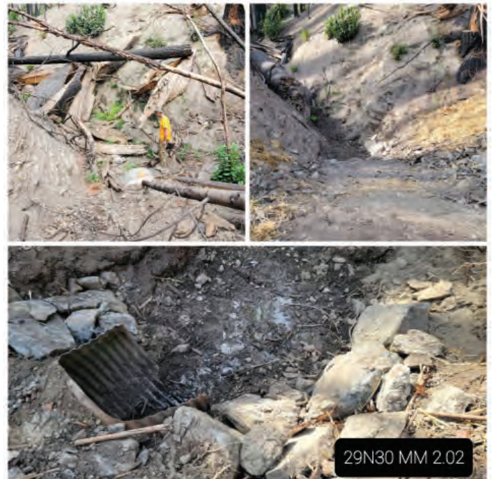
This stream crossing experienced high severity burn with many large trees near the culvert inlet. Trees were moved using an excavator and the existing culvert was reshaped to increase flow capacity and reduce plugging potential.
