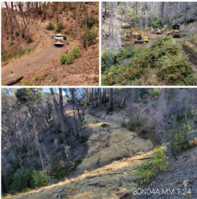
Before, during and after the road decommissioning project in the Wilson Creek Watershed near Wildwood.
