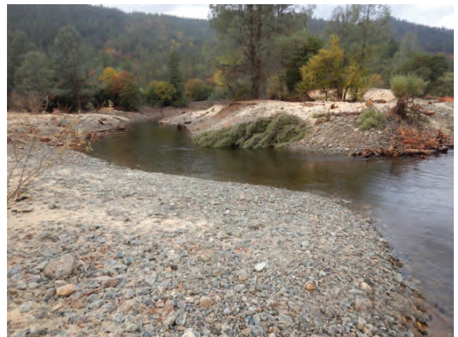
Figure 2. One of the three inlets constructed for the new side channel on river left at Chapman Ranch
