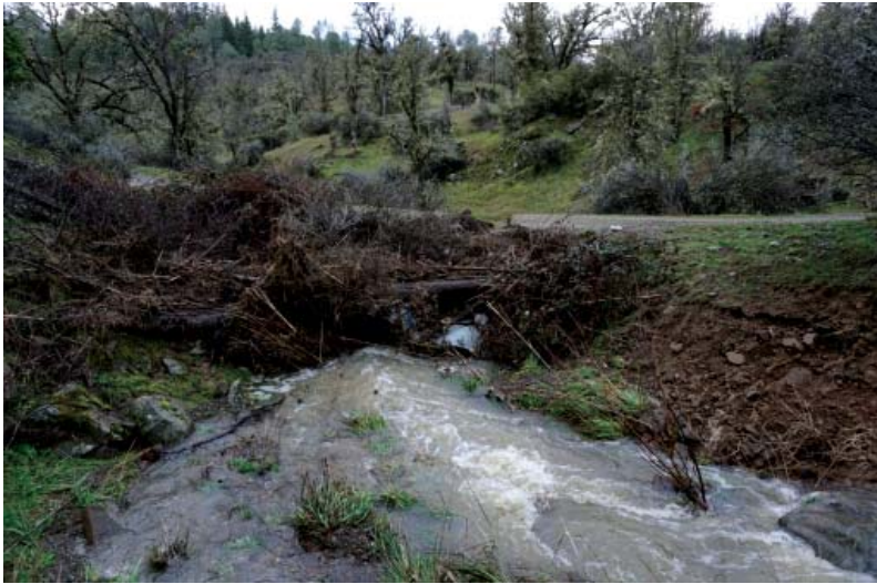
Culvert inlets following large rain event.
