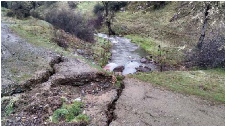
Culvert outlets after significant storm damage - early February 2015.
