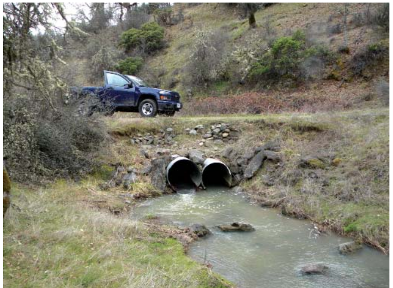
Pre-storm conditions in Browns Creek on private culvert.
