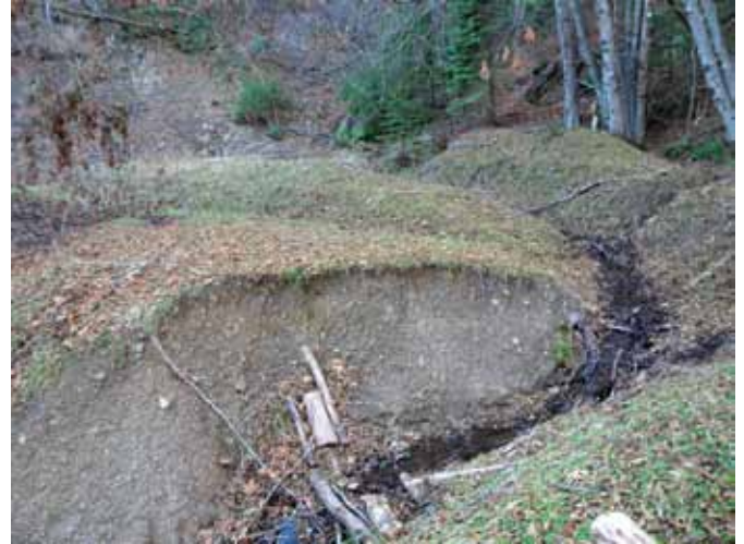
This road was constructed with no culvert pipe to let the water pass. Therefore the stream has cut down through the road fill, eroding the fill and contributing sediment pollution to the stream.
